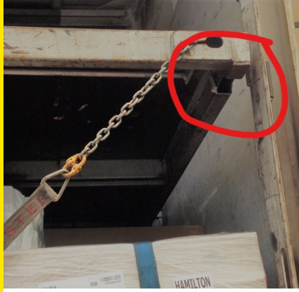
This image shows a mezz floor worn away where a support hook should be located.
