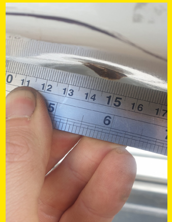
Boom damage impact
