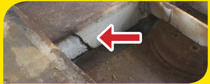
Structural cracks on a cross-member in the skid plate/kingpin assembly of a refrigerated trailer (found after the flooring was removed to reveal an internal chamber).
