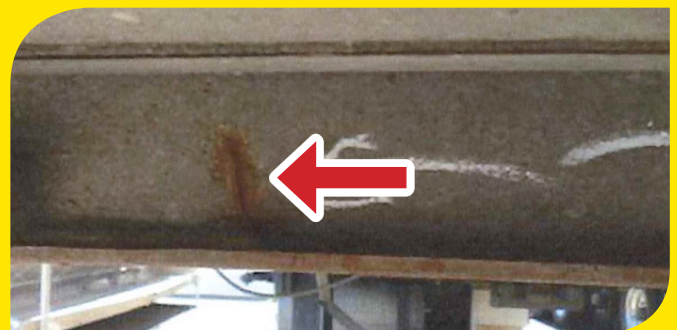
Major external crack - The unit must be removed from service.
