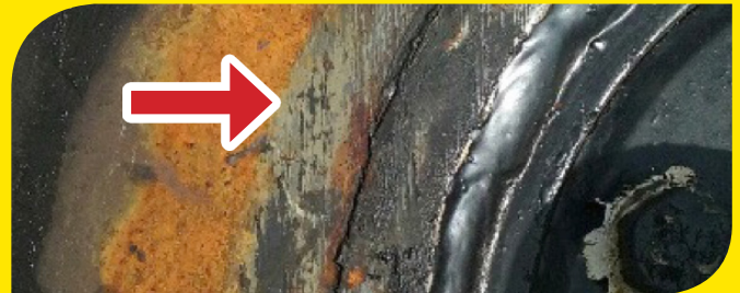
Failure of the internal cross members can lead to externally-visible cracks around the welds between the kingpin retention plate and the skid plate.
